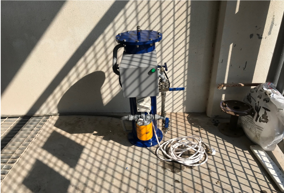
Fig 1.1 DryTrans TR5 Installation at Dewa Power Plant, Jebel Ali, UAE
