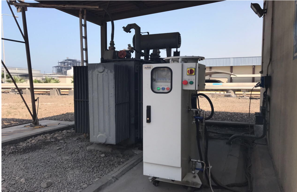
Fig 1.2 DryTrans MMS90 Installation at DUBAL Plant, Jabel Ali, UAE
