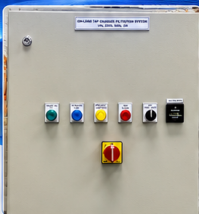
TRTC SYSTEM – FRONT VIEW
