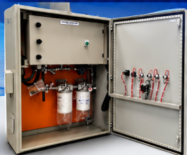
TRTC SYSTEM – INTERNAL VIEW
